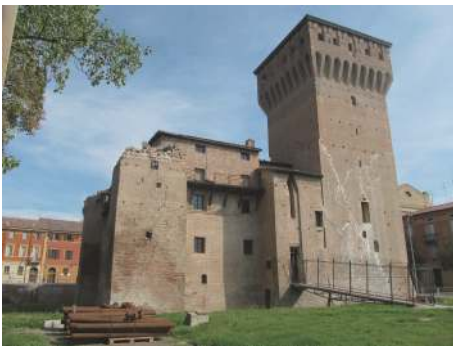
Fig. 2 Finale Emilia castle damaged by the earthquake
