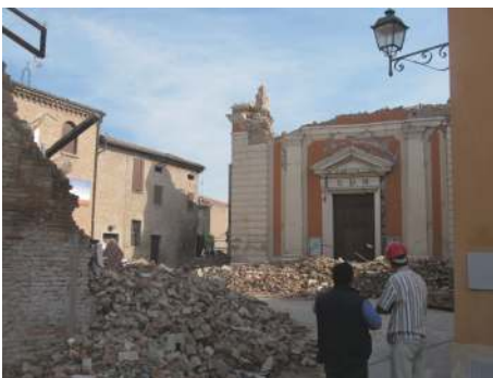
Fig. 3 One of the 296 churches damaged by the earthquake as seen in October 2012, five months after the main earthquakes, Cavezzo, Modena
